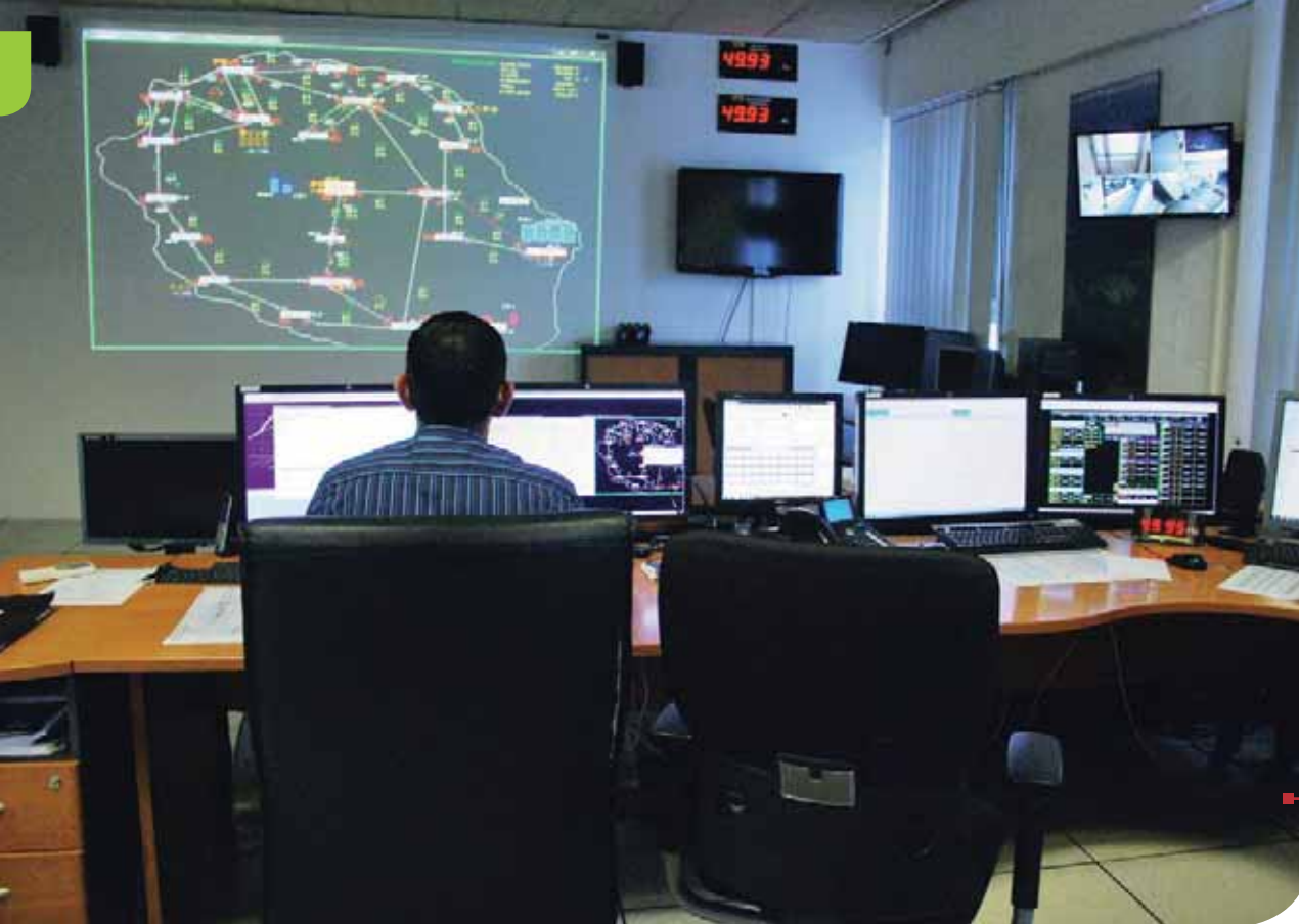
EDF DISPATCHING CENTRE IN SAINT-DENIS IN RÉUNION (VISIT OF CRE, OCTOBER 2014). © CRE
