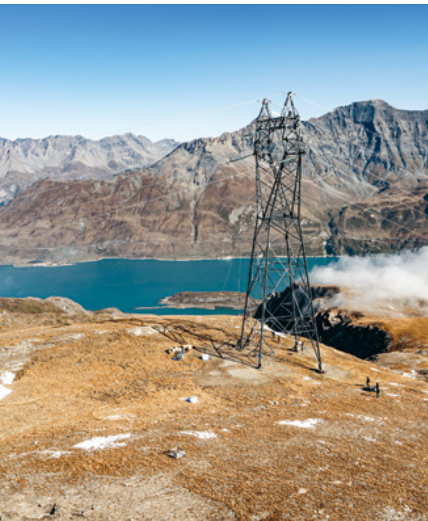
The 400,000-volt line linking Villarodin, near Modane, in Savoie, with Venaus, near Turin, Italy. It is one of the four strategic lines between France and Italy. © Seignette Lafontan
