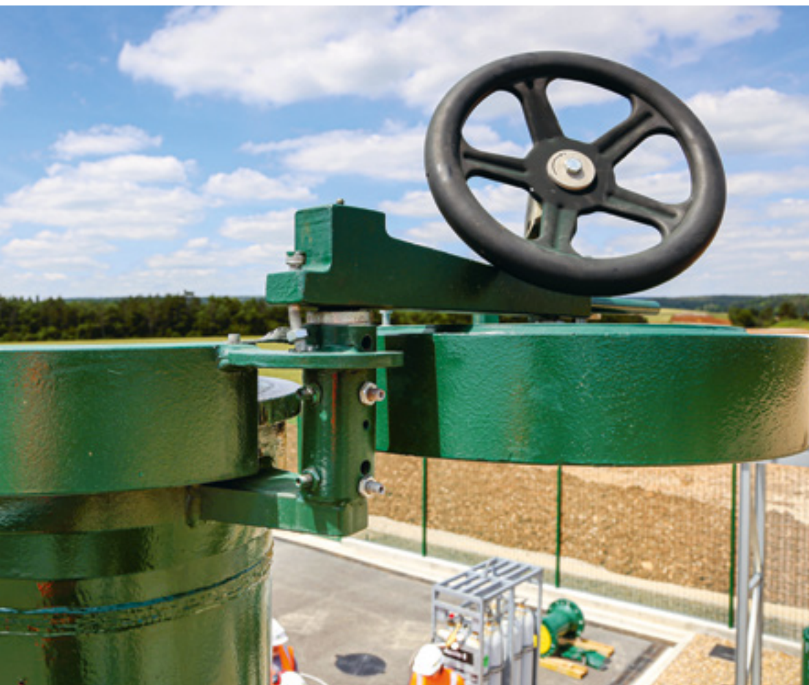
Switching station. © GRTgaz/AGENCE COMAIR
