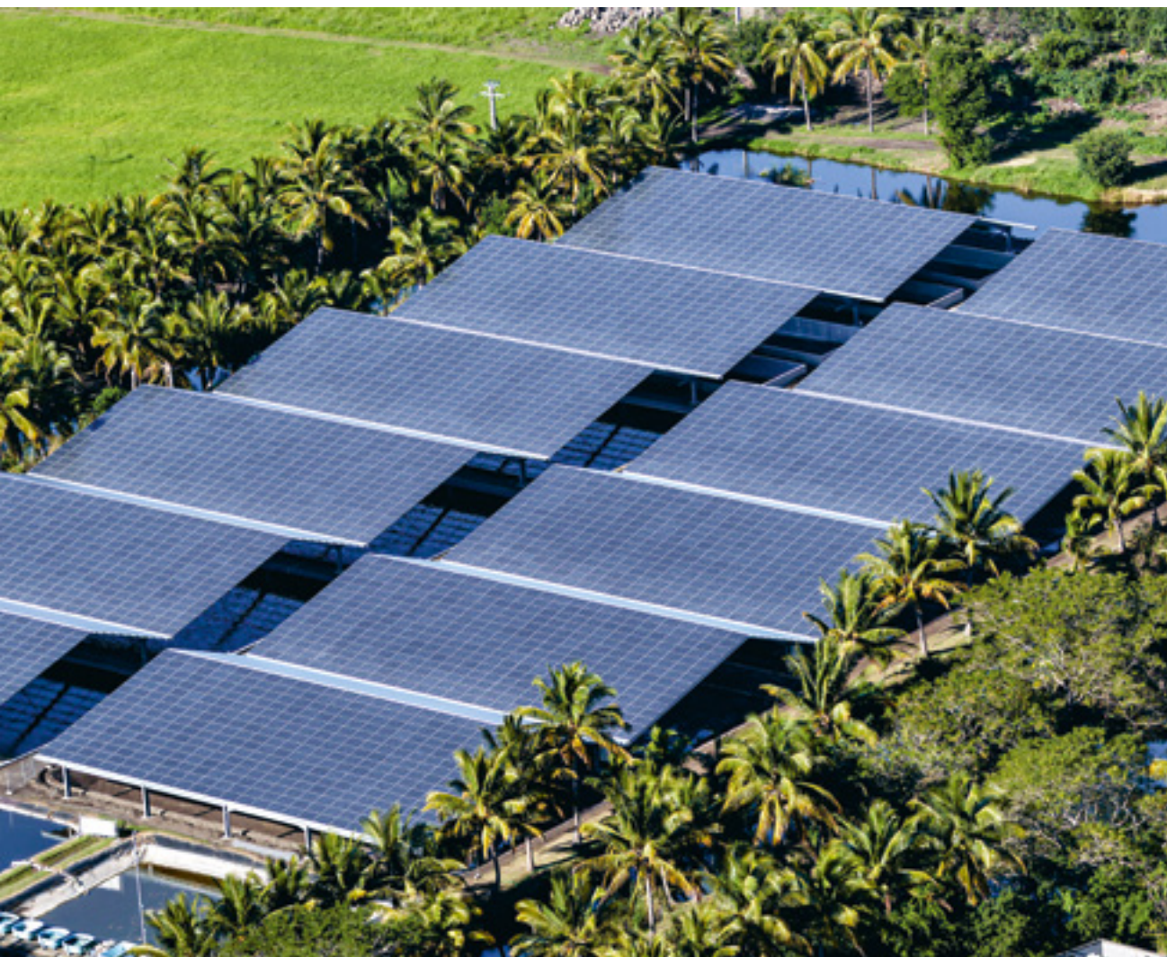
Photovoltaic park L'Étang-Salé in Réunion. © CRE
